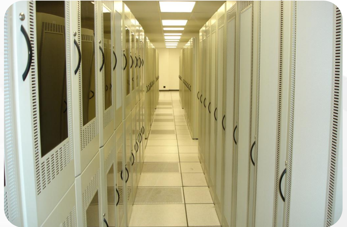
Datacenter 1: St. Paul, Minnesota
