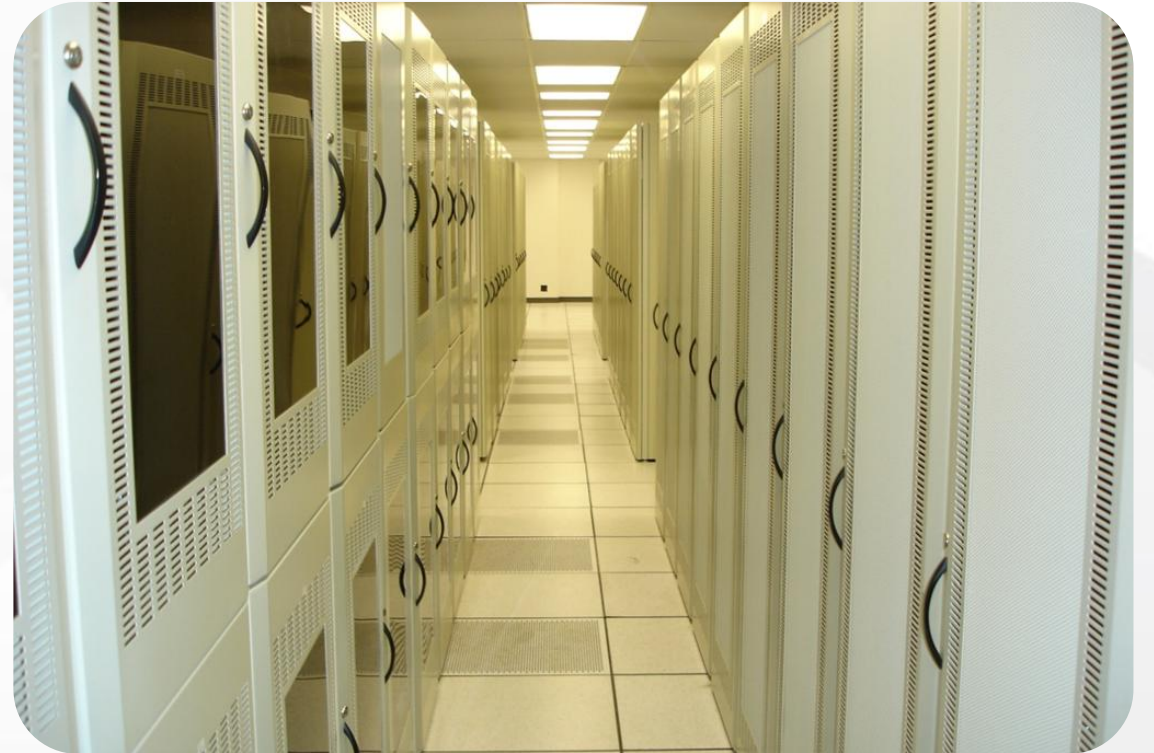
Datacenter 1: St. Paul, Minnesota
